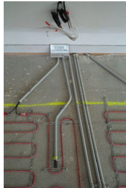
Locate sensor probe conduit central between cable runs for accurate temperature control.
